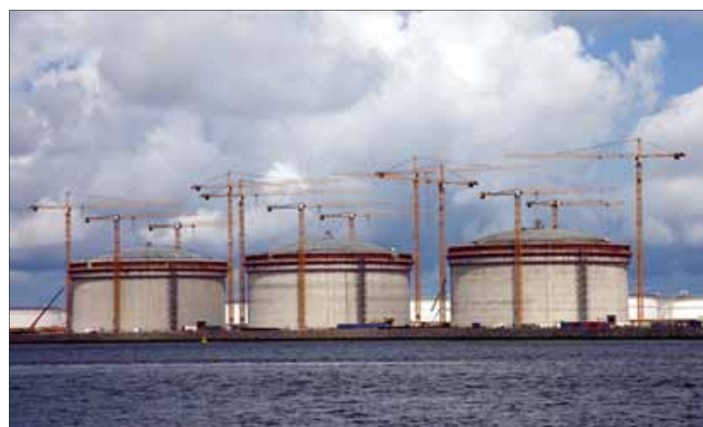
Gasunie and Vopak are jointly constructing the Gate terminal in Rotterdam, and the companies want to explore the possibilities for creating a CO 2 distribution hub
