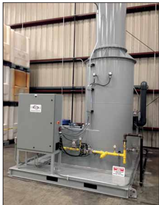
Hoover has installed thermo oxidiser units at its Scott and Houston sites
