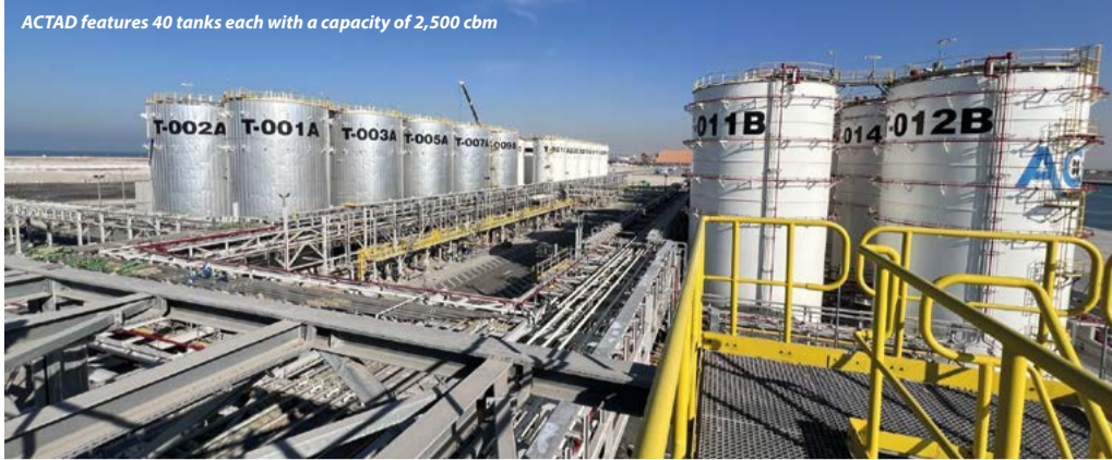
ACTAD features 40 tanks each with a capacity of 2,500 cbm
